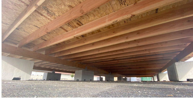
Figure 3.2: Photograph of support assembly for each structure. From the top down, this included the subfloor, floor joists, support beams, and concrete piers.
