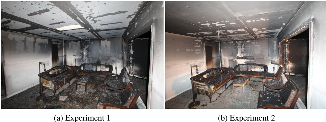
Figure 13: Post-suppression comparison of living room area of origin, with closed door.
