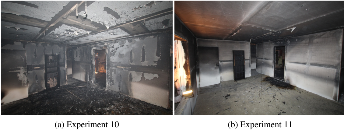
Figure 6.35: Post-suppression comparison of living room between kitchen room area of origin and open door.
