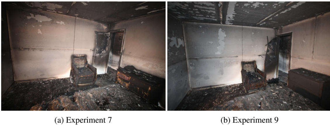
Figure 6.44: Post-suppression comparison of bedroom 1 opposite the area of origin with closed door.
