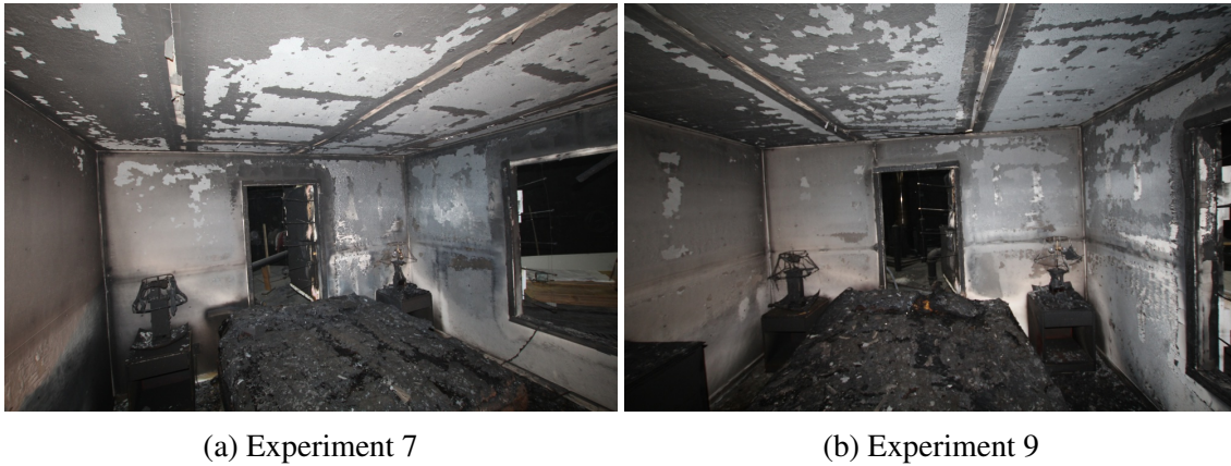
Figure 6.42: Post-suppression comparison of bedroom 1 area of origin with a closed door.
