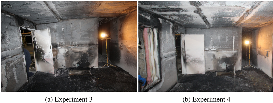
Figure 6.18: Post-overhaul comparison of living room wall opposite the area of origin and adjacent to front door with open door.
