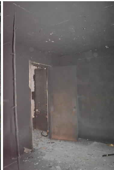
(e) Exp. 8 Open Front Door & Family Room Window
