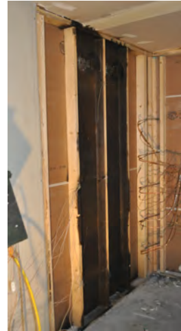
(b) Single Switch & Outlet Rear Overall
