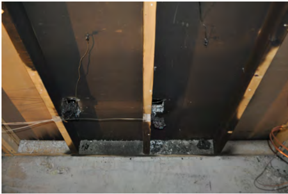
(c) Single Switch & Outlet Rear Bottom
