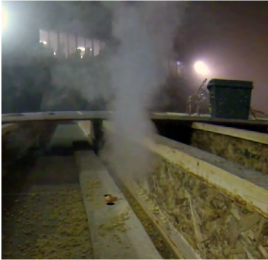
(a) Stud Bay Exhaust No-Fan
