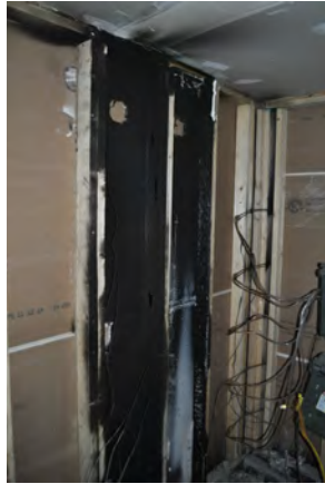
(a) Double Switch & Outlet Rear Overall
