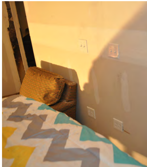
(b) Double Outlet and Switch Front
