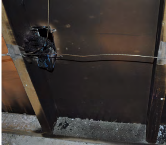
(a) Single Switch & Outlet Post Fire Rear
