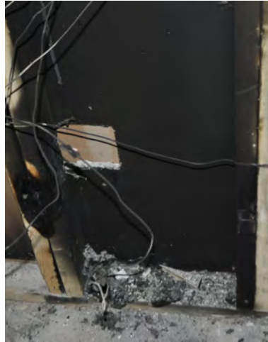
(b) Double Switch & Outlet Post Fire Rear
