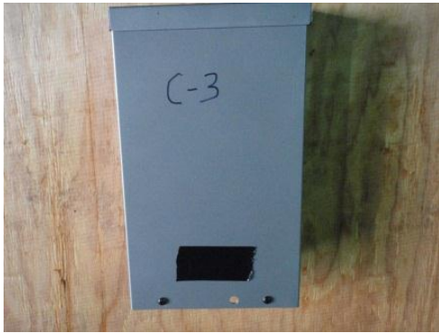
Figure 21 Combiner Box C3
