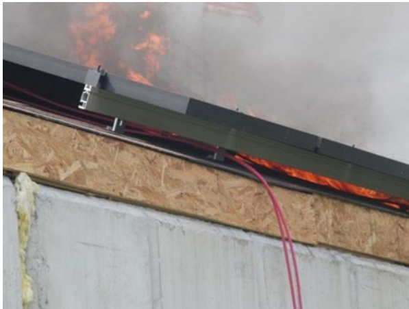
Figure 173 Fire propagating under modules
