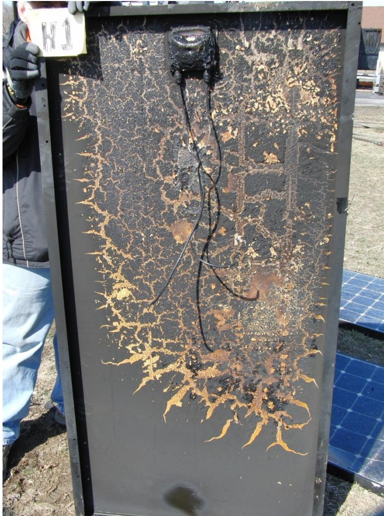
Figure 120 Module H1 – junction box burned, but still fully operational
