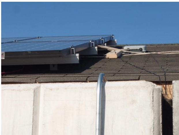
Figure 89 Modules mounted off roof / EMT to inverter
