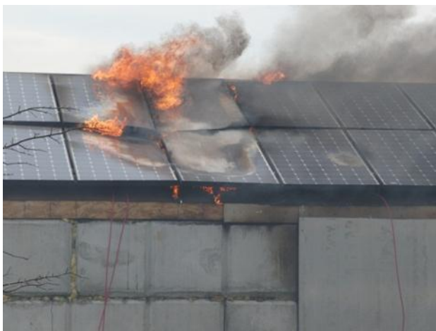
Figure 175 Modules sagging from heat
