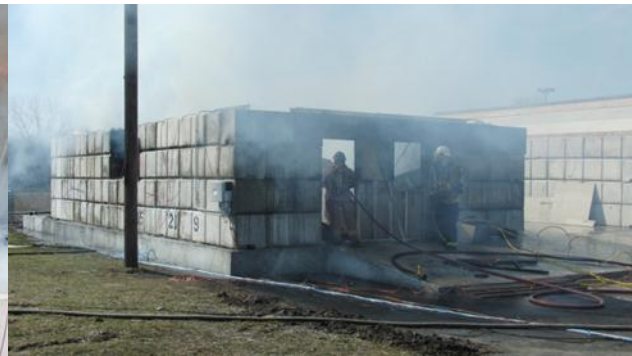
Figure 104 Roof collapsed -fire extinguished
