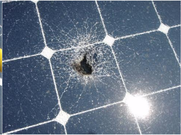
Figure 64 Resulting hole in module glass
