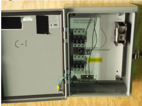
Figure 18 Combiner Box C1 Open
