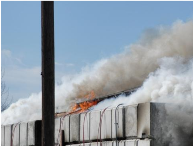
Figure 101 Open flames on roof
