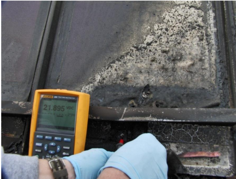
Figure 140 Full voltage measured at damaged laminate
