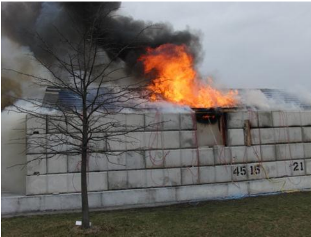
Figure 146 Solar shingles on fire
