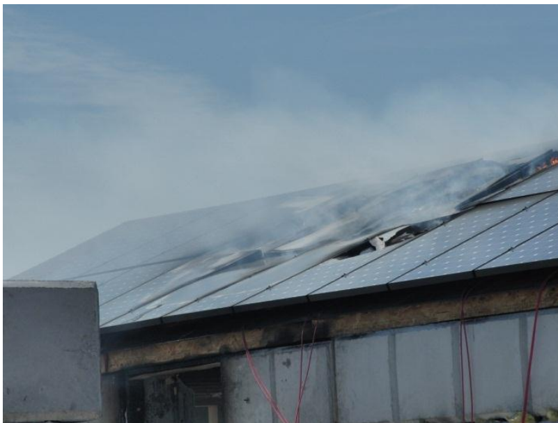
Figure 191 Broken glass and debris
