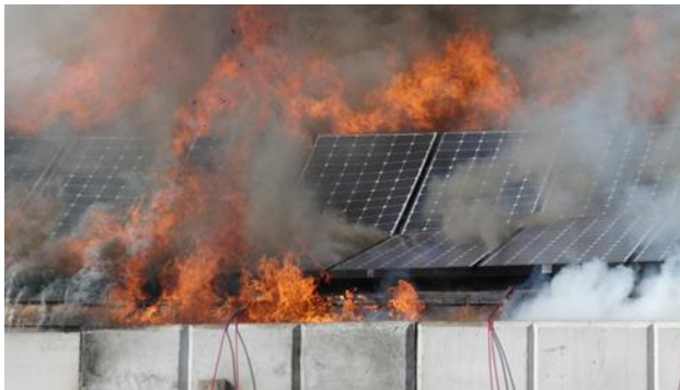
Figure 103 Roof and modules collapsing
