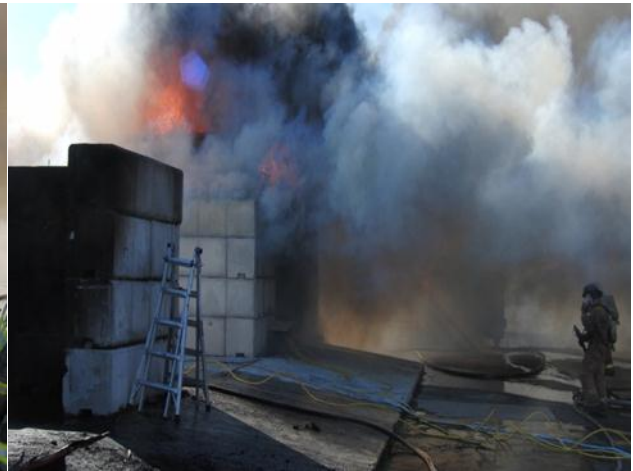
Figure 126 Roof and laminates collapsing
