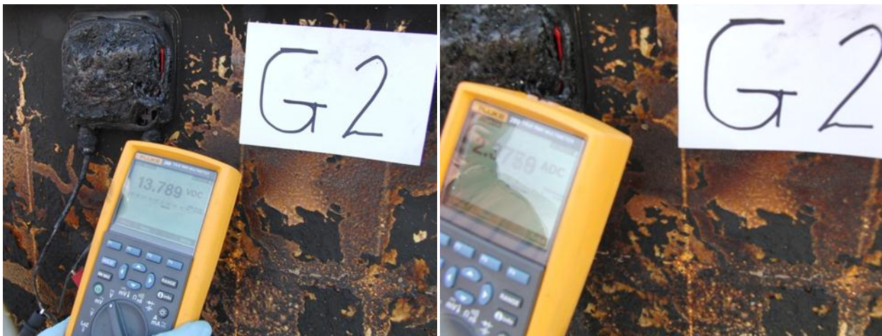
Figure 119 Module G2 – still producing voltage and current
