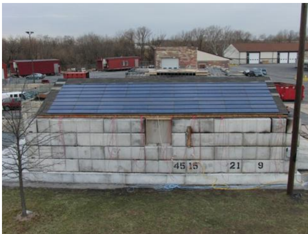
Figure 142 Pre-test conditions with shingles
