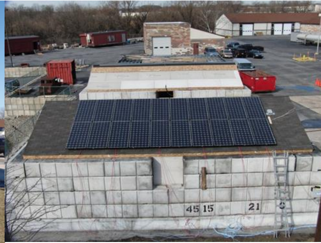
Figure 86 Framed module array from above
