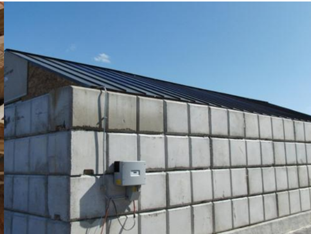
Figure 93 Inverter/disconnect near ground
