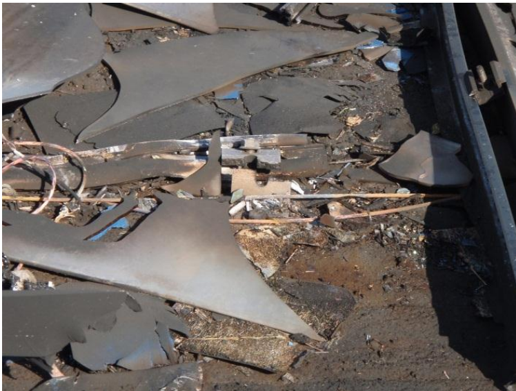
Figure 197 Bare Conductors in Debris on Roof
