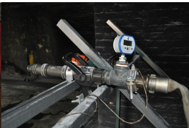
Figure 7 Electrical connection to hose fitting
