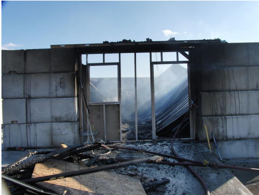
Figure 127 Collapsed roof and laminates
