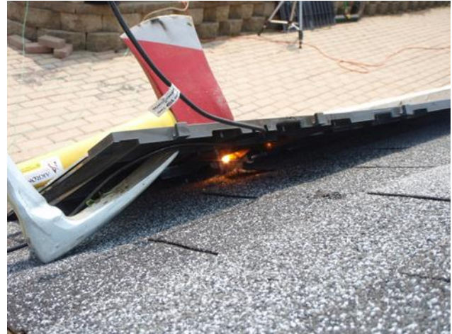
Figure 69 Resulting arcing and flame
