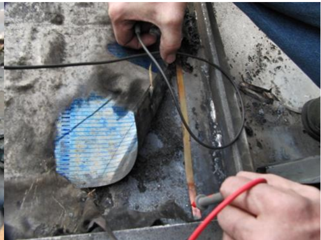
Figure 139 - Exposed bare live bus
