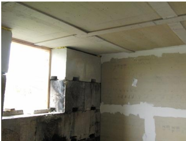
Figure 162 Confined ignition space in bunker
