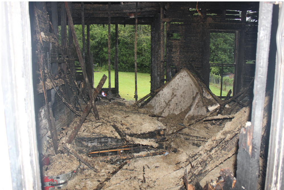
Figure 4.8: Photograph of the bedroom from the entry door looking toward side C.
