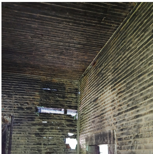
Figure 4.3: Photograph of the interior finish of the walls and ceiling of the structure. This image was taken in the living room but is representative of the bead board that formed the interior surface of the walls and ceiling in the kitchen and bedroom before the fire.
