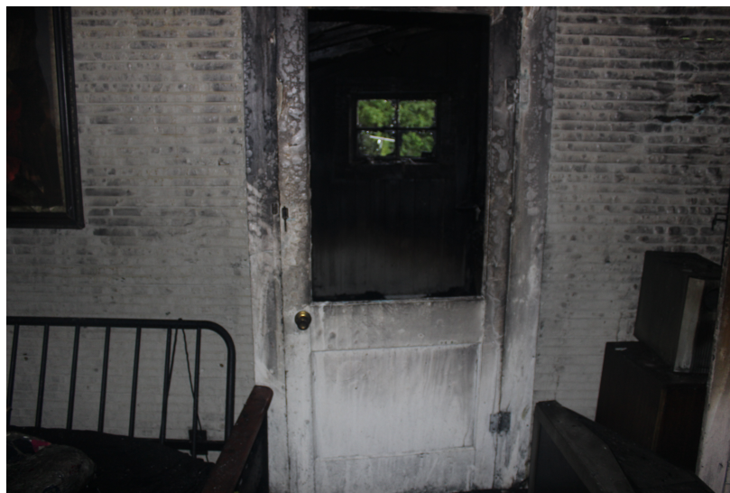
Figure 4.11: Photograph of the door, which leads to the hallway between the bathroom and the kitchen. Photo taken from the living room looking toward the rear of the structure.
