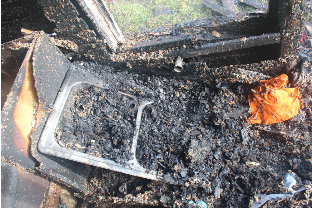
Figure 4.14: Photograph of the sink cabinet below the window on the side C wall.
