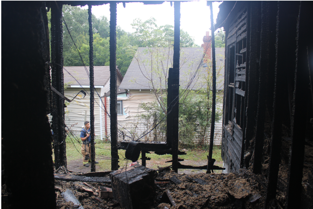
Figure 4.15: Photograph of the kitchen side D wall. Remains of the window framing for the sill can be seen.
