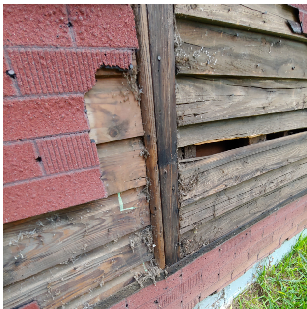
Figure 4.2: Photograph of an exterior wall of the structure showing the asphalt siding was installed over the wood siding.
